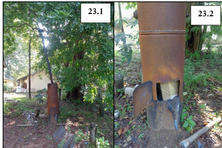
Burner by which sharps are combusted
