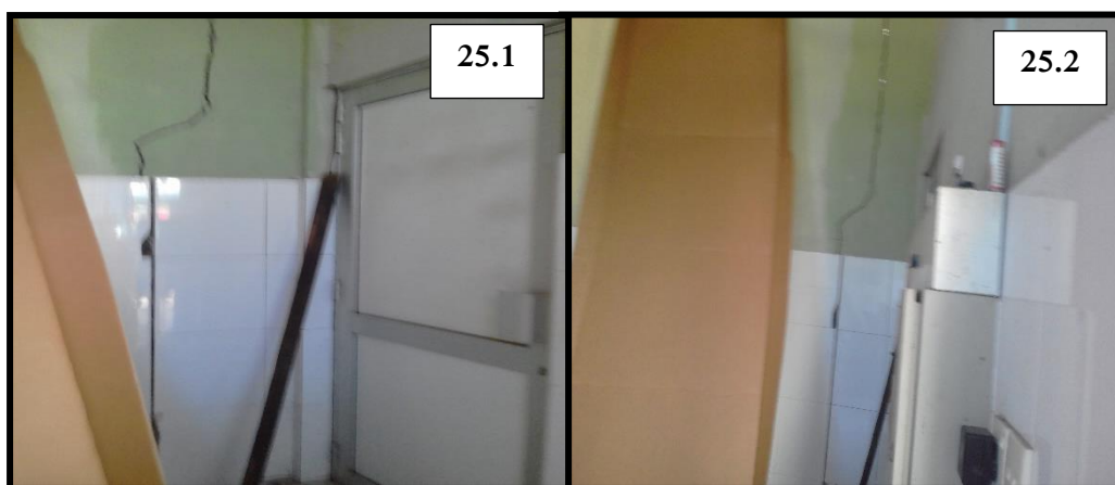
The cracked wall
